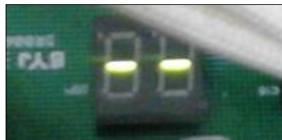
PIC 4 :Main board LED when power on and unit standby.
